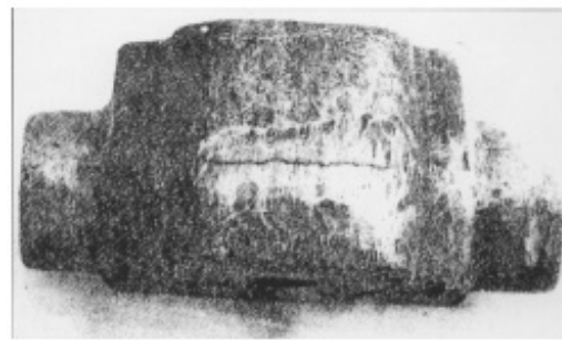
Flash line crack
